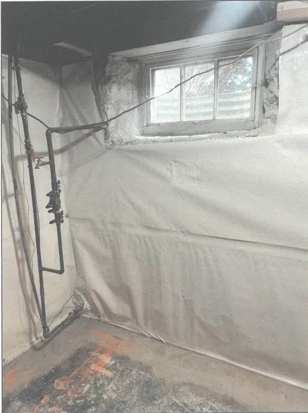
Picture 1 – Current Basement: Window in the Basement that would require an Egress Window.
