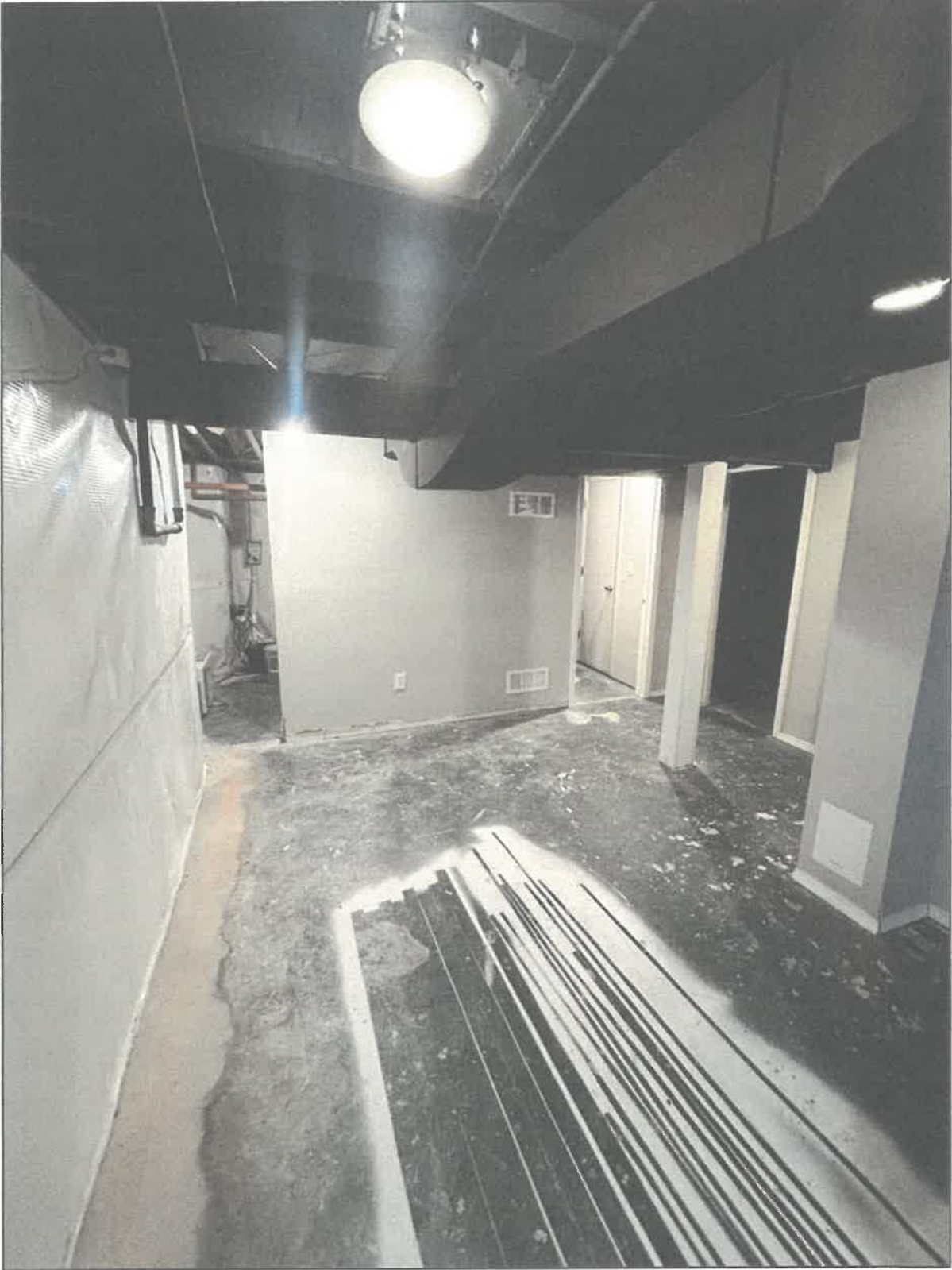
Picture 4: Showing existing basement layout, vapor barrier walls, unfinished floor and ceiling.
