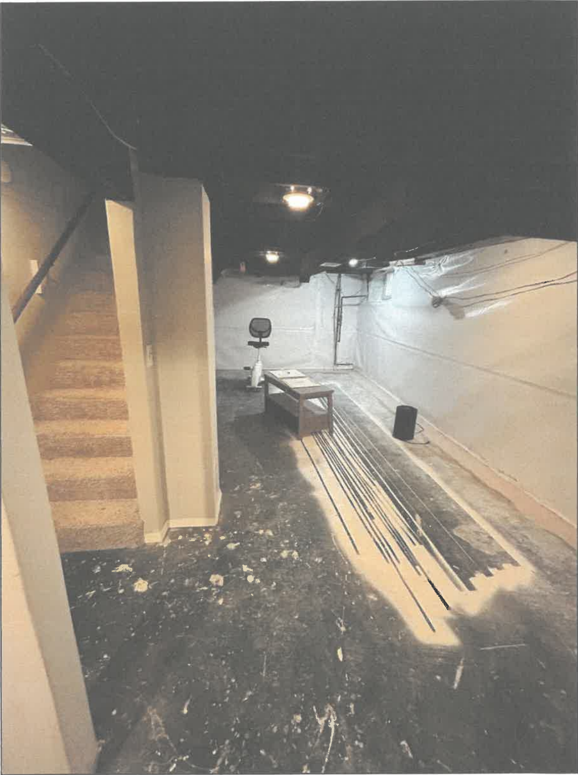
Picture 2 - Current Basement: showing reasoning for new walls and framing of electrical.
